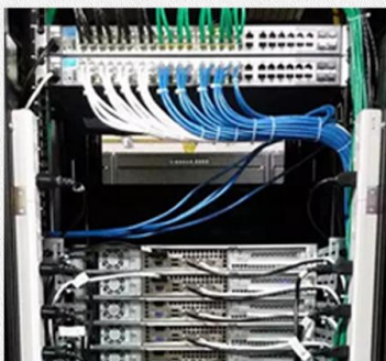
Computer room wiring
