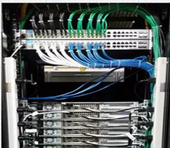
Computer room wiring
